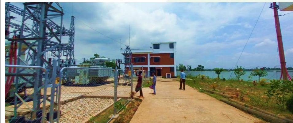
Name: 33/11 KV Sub-Station Location: Kaliakoir-6, Customer: EnergyPac
