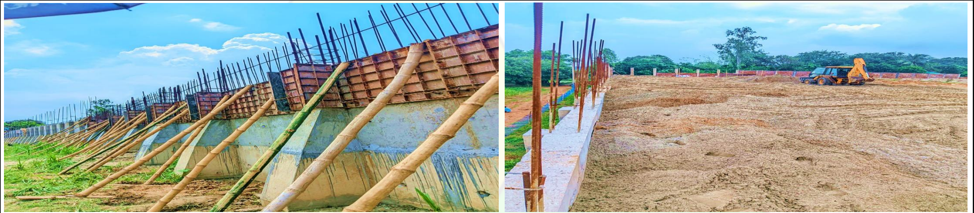
Name: 230/33 KV GIS Sub-Station Location: Kashimpur, Gazipur Customer: EnergyPac
