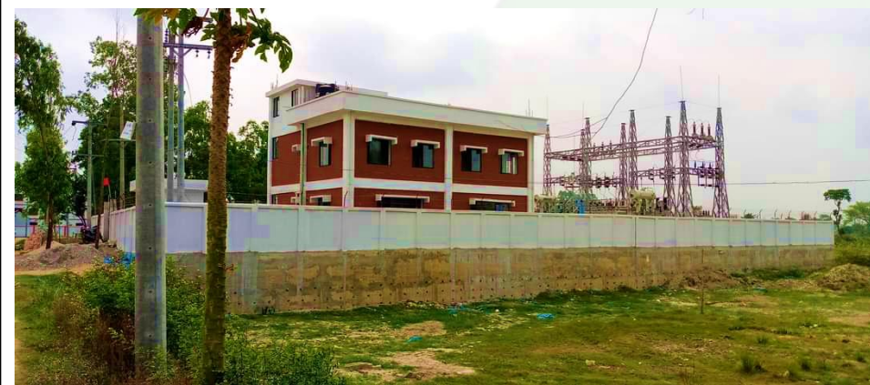
Name: 33/11 KV Sub-Station Location: Mirzapur-8, Customer: EnergyPac
